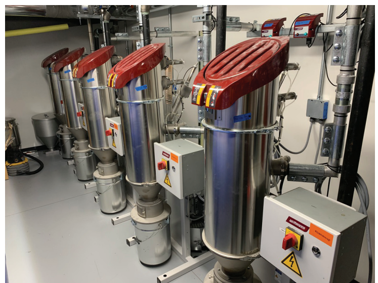
Five WITTMANN XMB vacuum pumps in their own dedicated room
