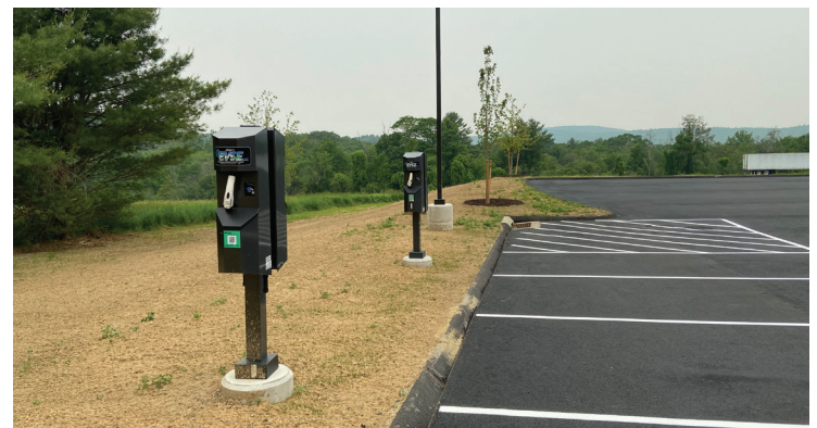
Plant 1 New Electric Charging Stations
